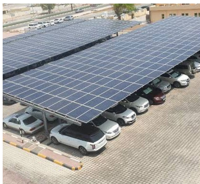
Figure 10: Solar carport at Ras Al Khaimah Municipality
