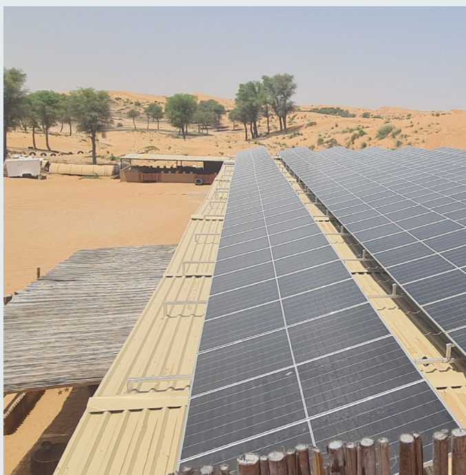
Figure 11: Solar installation at Bassata Desert Village camp
