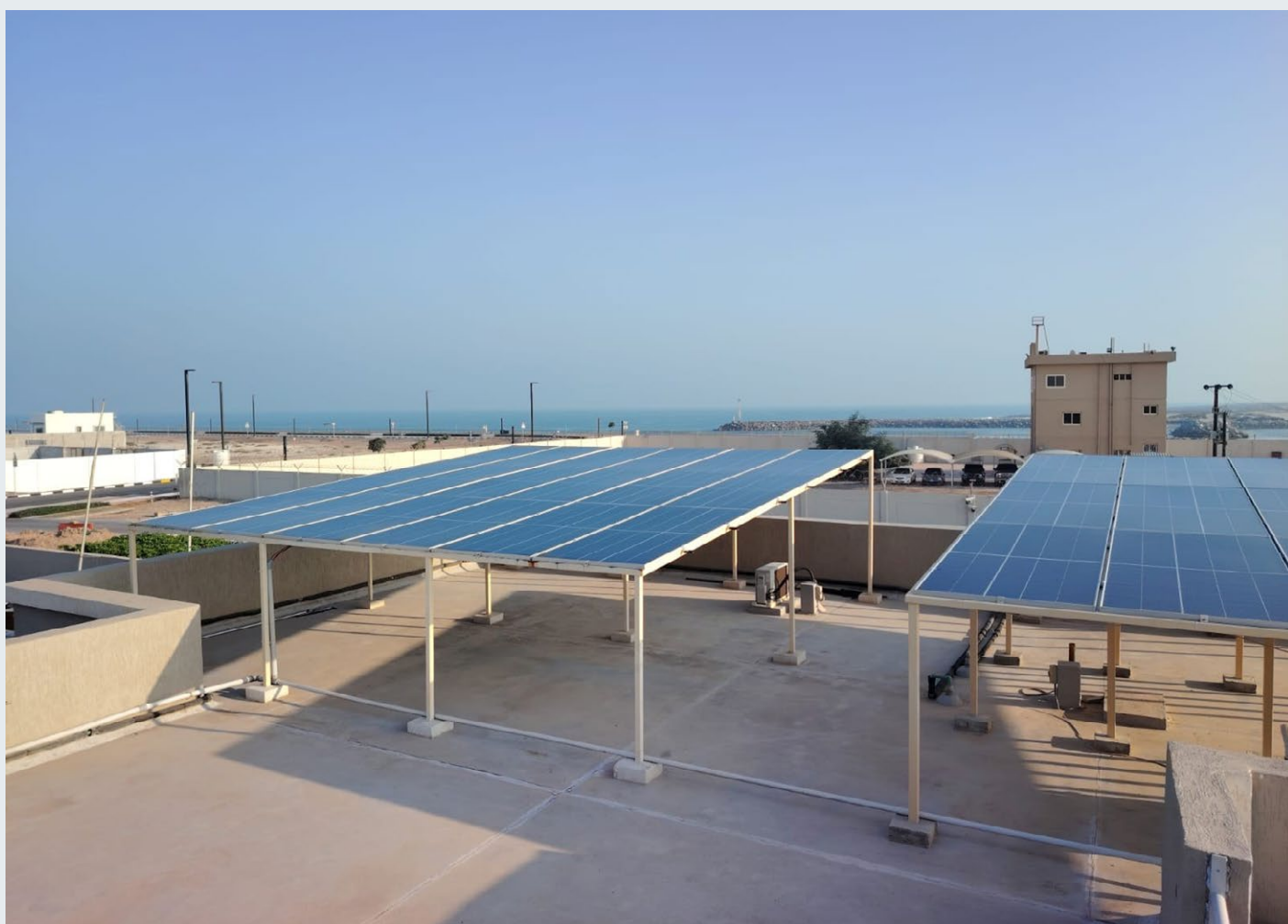
Figure 11: Solar installation at RAK Sailing Association
