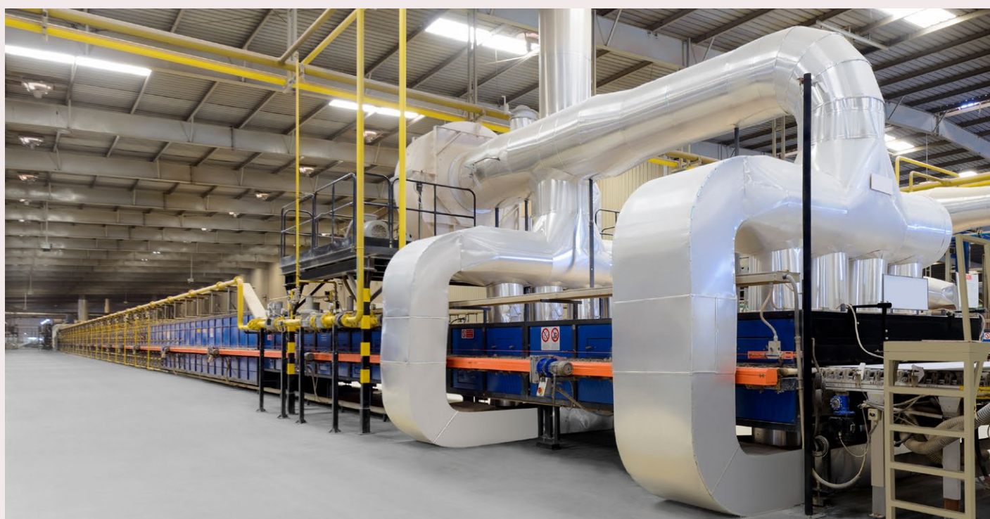
Figure 32: Waste heat recovery system at RAK Ceramics
