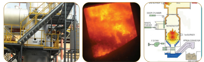
Figure 26: Medical waste incinerator in Ras Al Khaimah
